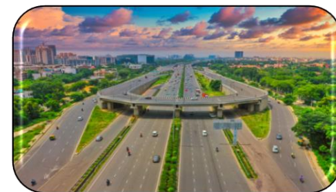
Delhi-Mumbai Expressway (Under construction, to reduce travel time between Delhi & Mumbai from 24 hours to 12 hours)
